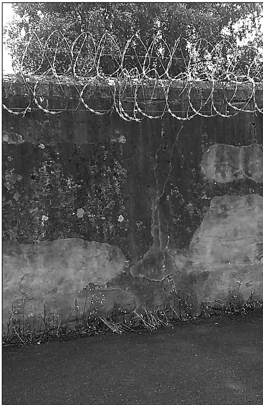
The wall at the Military Detention Barracks, Curragh Camp, where 7 men of the Rathbride Column were executed
